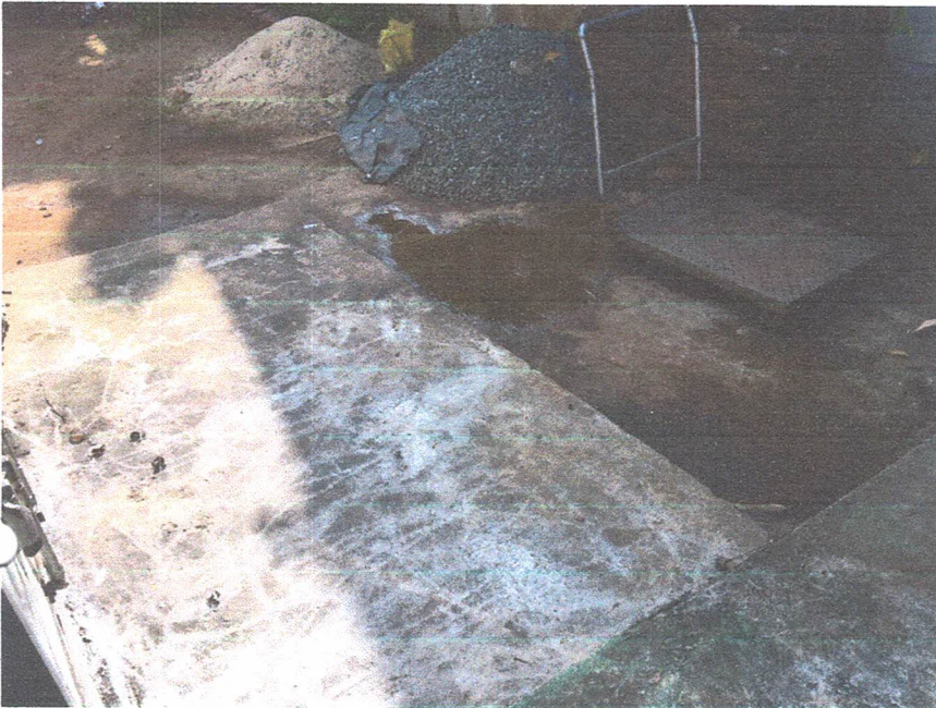
Water stagnated point near cold room
