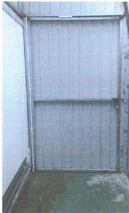
Door after cover gaps
