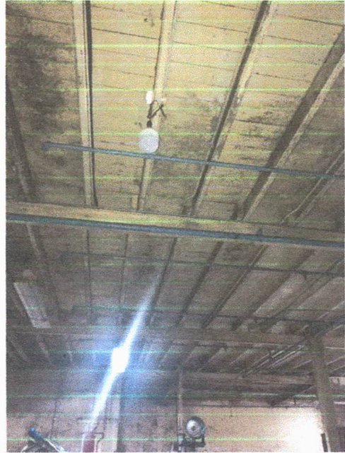
After replaced with LED bulb
