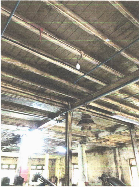
Uncovered glass bulb in rolling area
