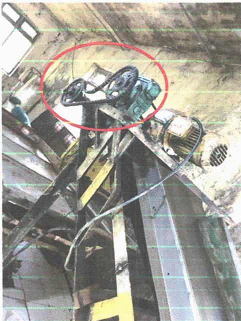
Uncovered motor chain
